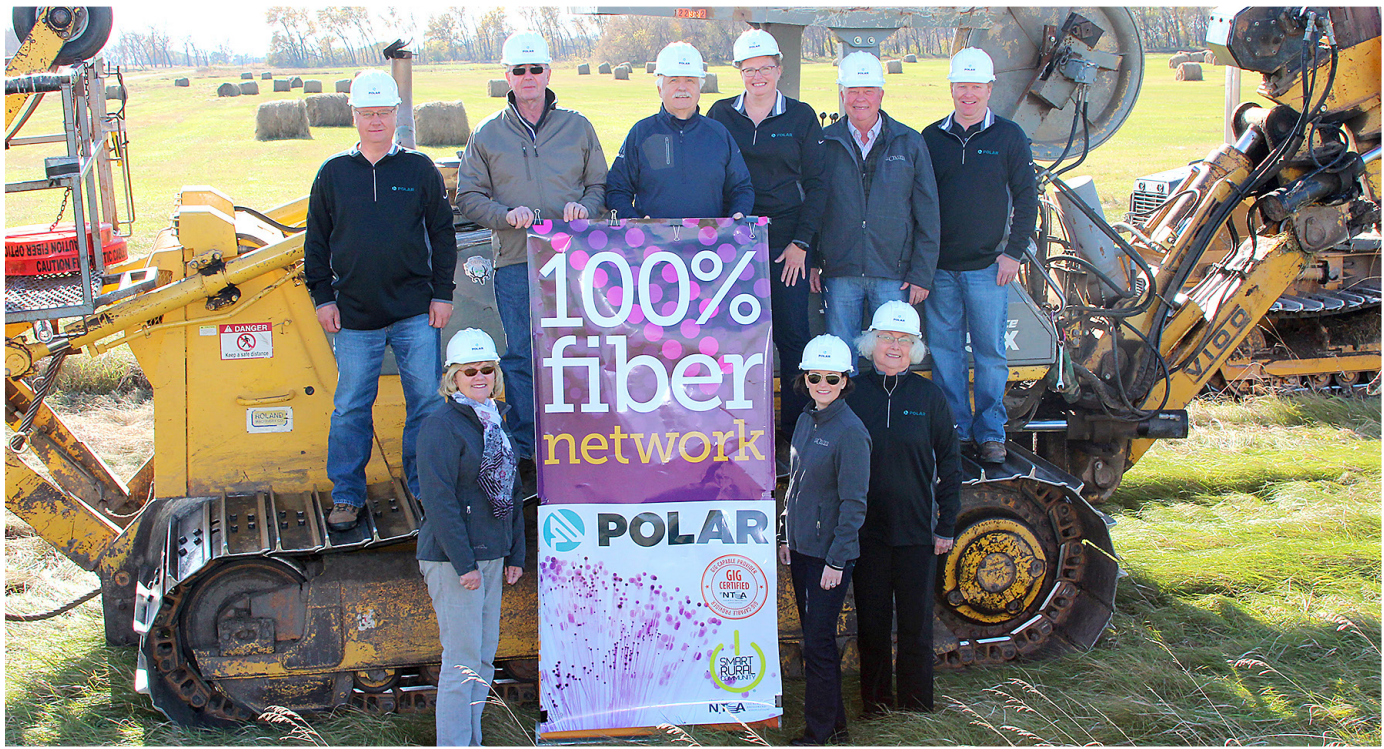
Polar Communications Board Members and CEO join the construction crew for the last mile of fiber plowed in the service area. Top Row - L to R: Brian Udby, President Ron Steinke, General Manager/CEO Dave Dunning, Lori Dahl, Jon McMillan, and Chris Nelson. Bottom Row - L to R: Cindy Hejl, Amber Meyer, and Beverly Jensen. Not Pictured: Joe Torgerson
